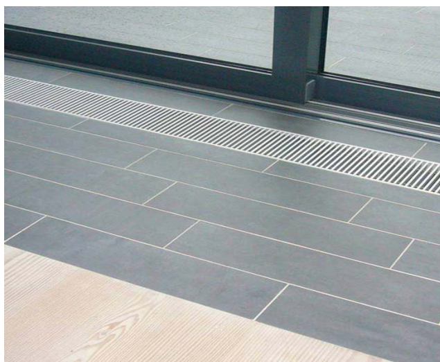
Perimeter floor heating
